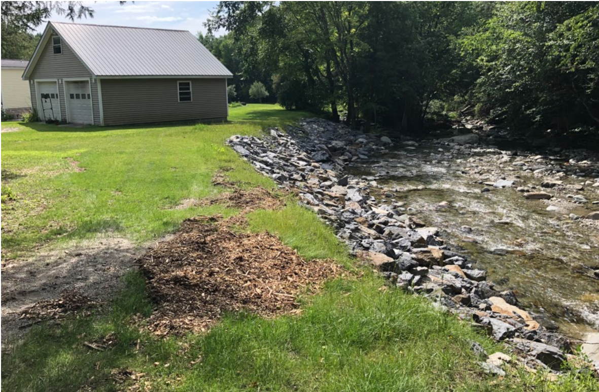
After EWP repairs, the streambank has been stabilized to prevent further bank erosion and danger to the buildings.
